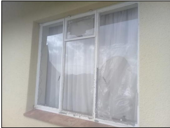
Figure 13: Broken window Da Gama Park
